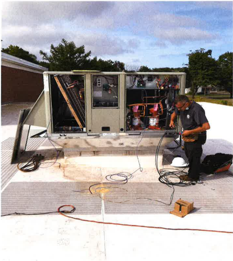
Newtown Middle School – New rooftop a/c unit, E-wing (in-house)
