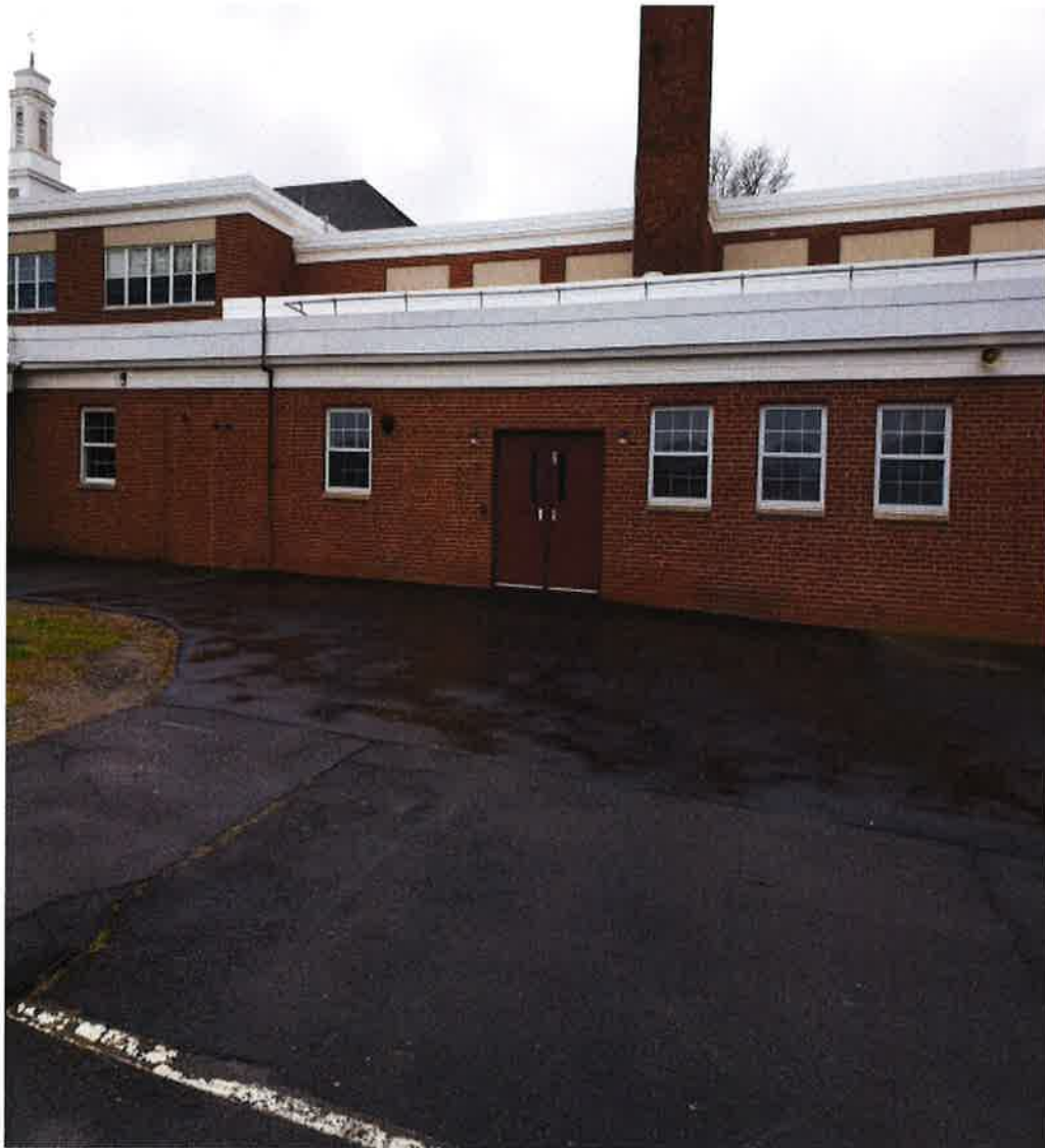
Newtown Middle School – Replace missing brick and repointed mortar joints
